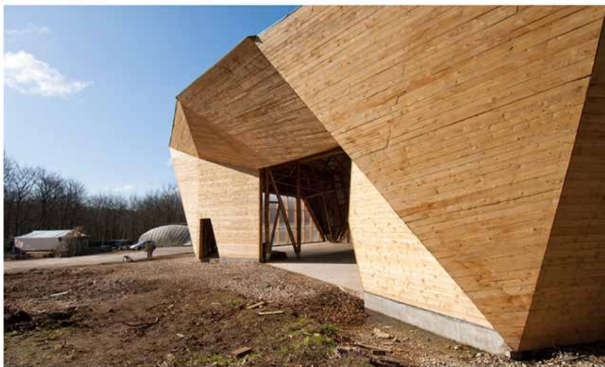
the structure sits on a concrete foundation that serves as the ideal floor for a multi-functional indoor/outdoor workshop image © valerie bennett
